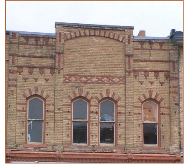
The gable and finial of the centre section is now missing, but the upper façade is still much as it once was.
