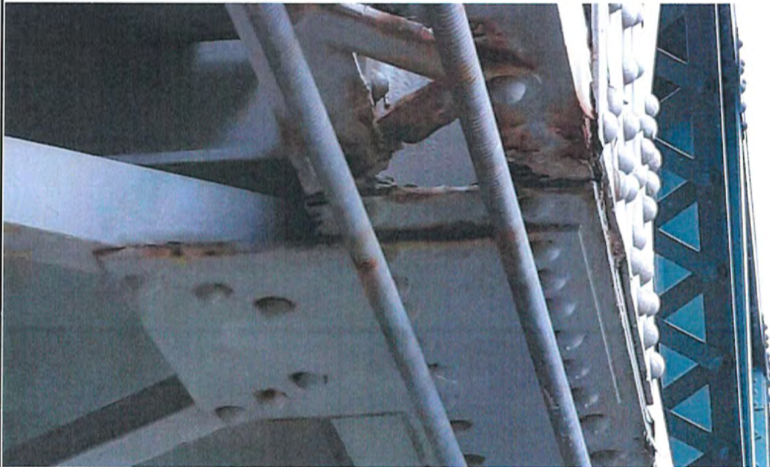
Bottom Chord Deterioration - East Truss
