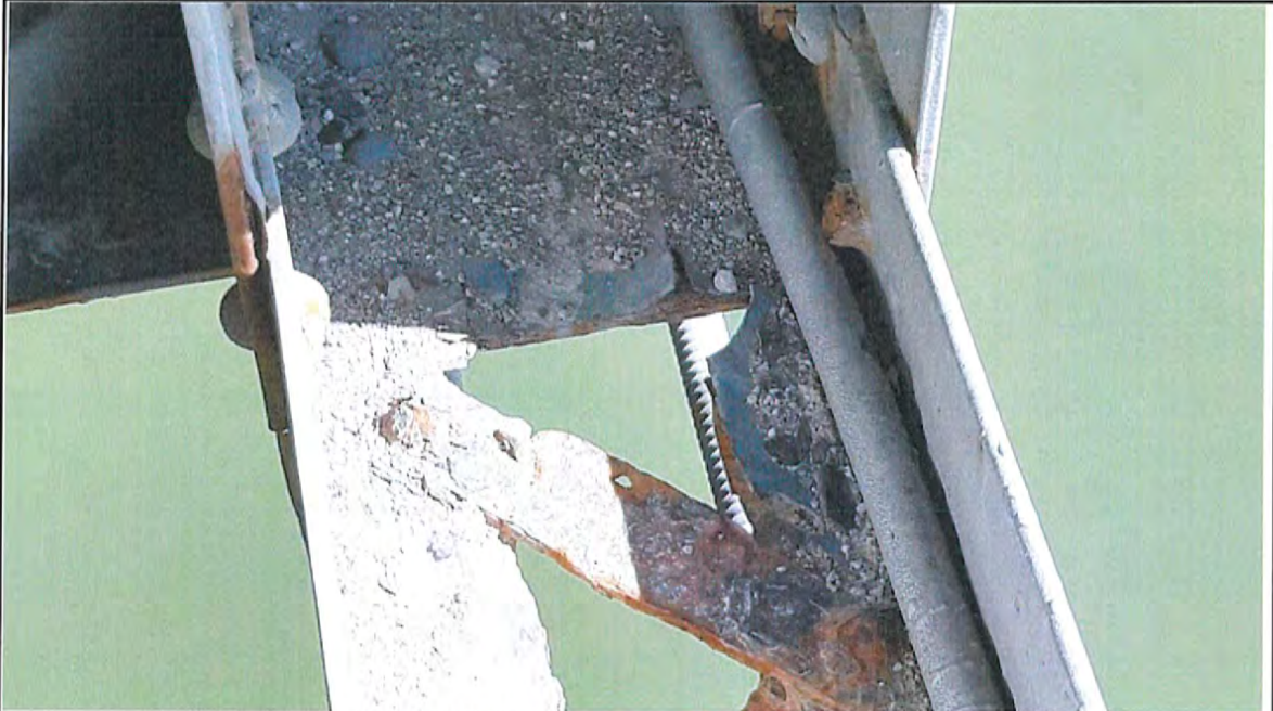
Bottom Chord Deterioration - East Truss
