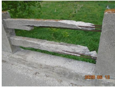
North Railing – Broken Rails
